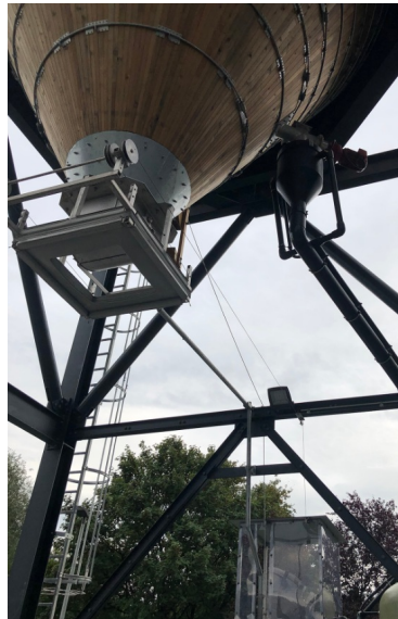
Automated brine system with storage tank
