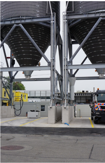
Brine generator with storage tank and control tank
