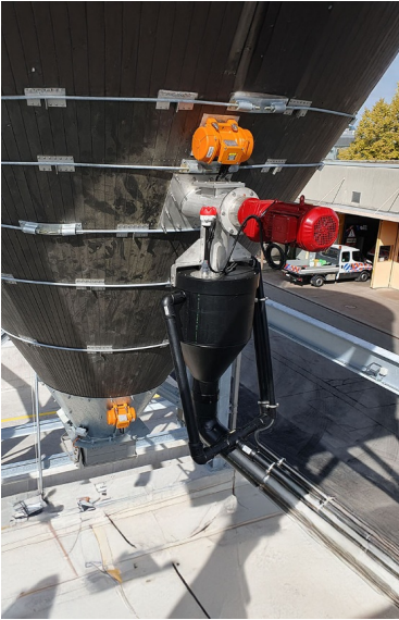
Brine tank system with control point
