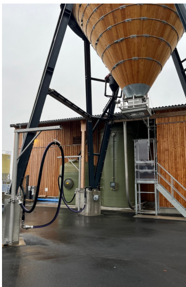
Brine fuelling station, operating platform and silo outlet with height-adjustable windsock
