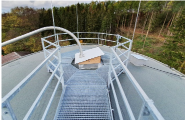
Brine filling station with control unit
