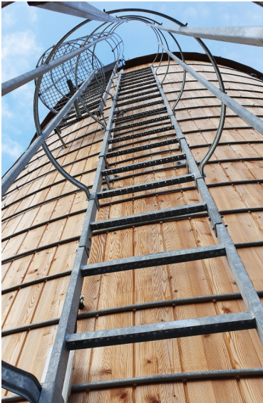
Access ladder of hot-dip galvanised steel
