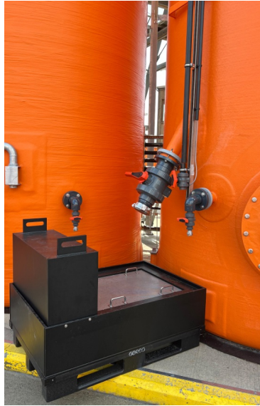
Soleanlage Percostrasse in Wien
